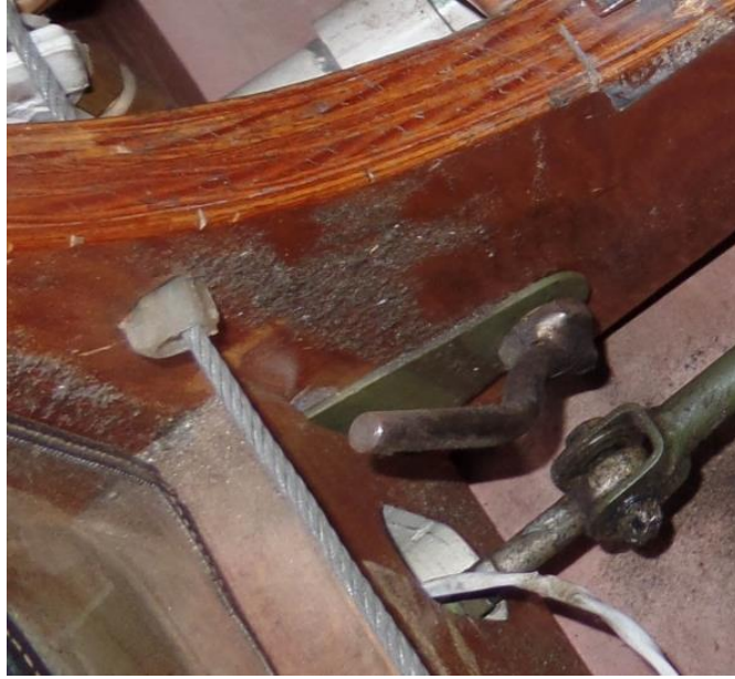
Figure 56: Rudder Cable Fairlead in Bulkhead
